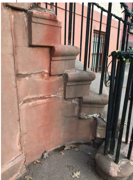
It is best to determine the reason for the damage and to eliminate that threat to the stone before making repairs.
