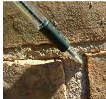
Soft mortar will shed granules of sand when scratched with a key or a pen.
