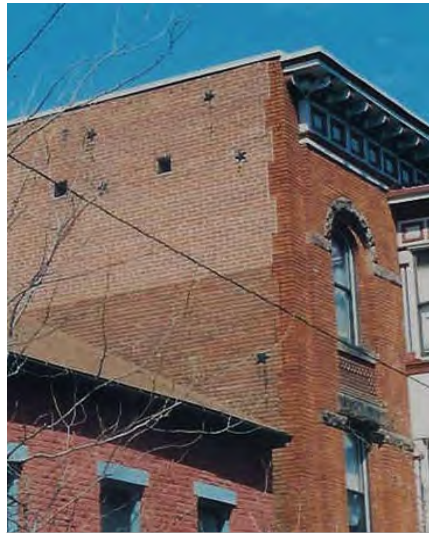
Poor quality repointing work is easy to spot. Inorganic pigments can be used to tint mortar so it matches the historic.
