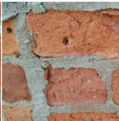
The use of hard mortar has caused the face of these bricks to spall.
