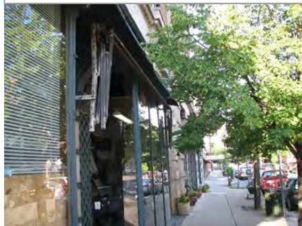
Proper pruning will assure that tree canopy does not interfere with building components or pedestrian safety
